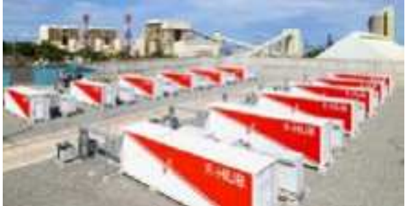
SMC has invested in battery storage facilities throughout the country to help ensure stable, reliable electricity while supporting the integration of more renewable capacities to the grid.
